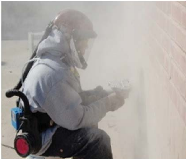
Figure 39. Tuck-pointing without controls
