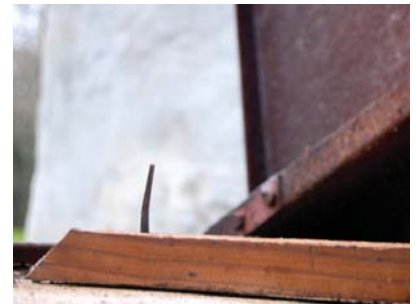
Figure 22. Nail protruding from wood.
