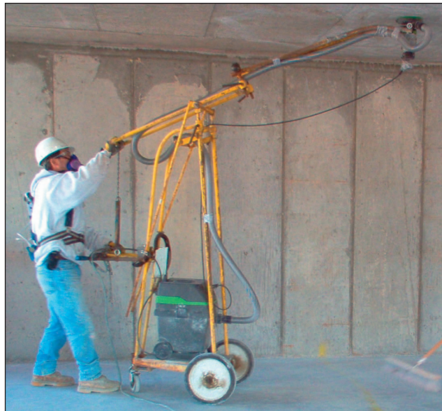
A cement finisher wears a respirator while testing dust control on an overhead grinder.
